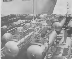
THE DISCOVERY of water in the feed, top photo, slightly slowed down "come up" of south unit. Treater J. B. Thijssen, second photo, tests feed for caustic. Final check on caustic circulator rate recorder, third photo, is made by Instrument Foreman N. J. Smith. The 200,000 electrical coalescers replaced existing capacity in Light Oils Finishing.
